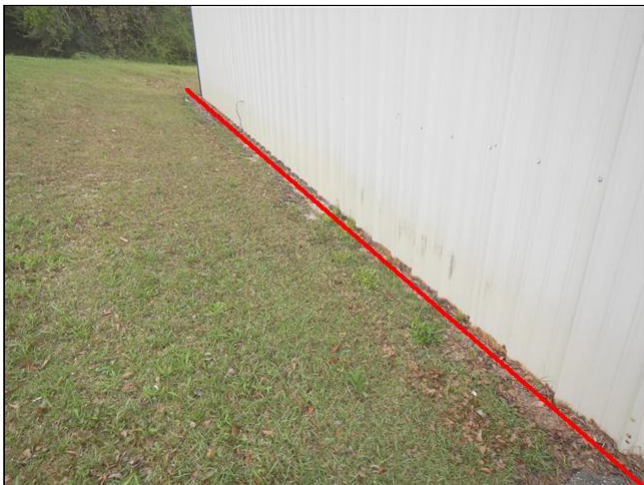
Item 3 - Item 1(Picture) The soil on this side of the building is higher than the floor. This is allowing water to enter into the building. The soil needs to be four to six inches below the floor.
