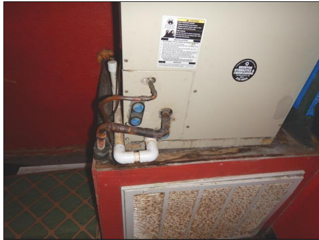
7.2 Item 2(Picture) The platform for the air handler has water damage.
