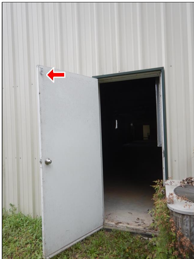
2.1 Item 1(Picture) The door lock for this door does not work. It has to be secured with a bolt at the top of the door.
