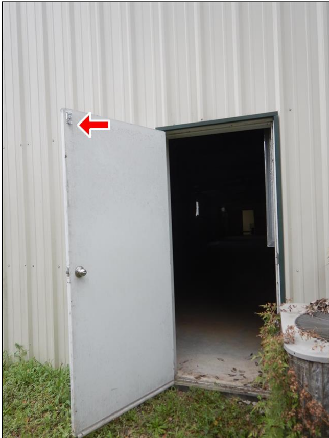
Item 2 - Item 1(Picture) The door lock for this door does not work. It has to be secured with a bolt at the top of the door.
