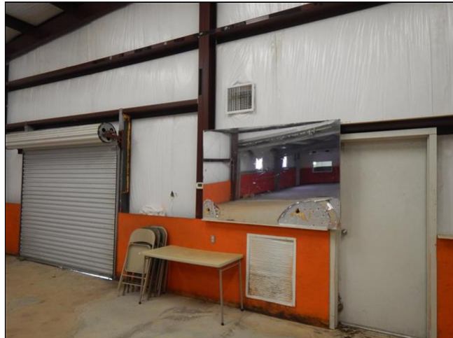
7.3 Item 2(Picture) The HVAC for the gym does not have duct work.
