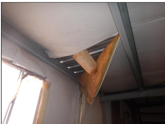
8.0 Item 1(Picture) There are several areas where the insulation is loose.
