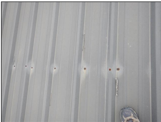
1.0 Item 1(Picture) The screws for the roofing are corroded with rust. They are recommended to be replaced.
