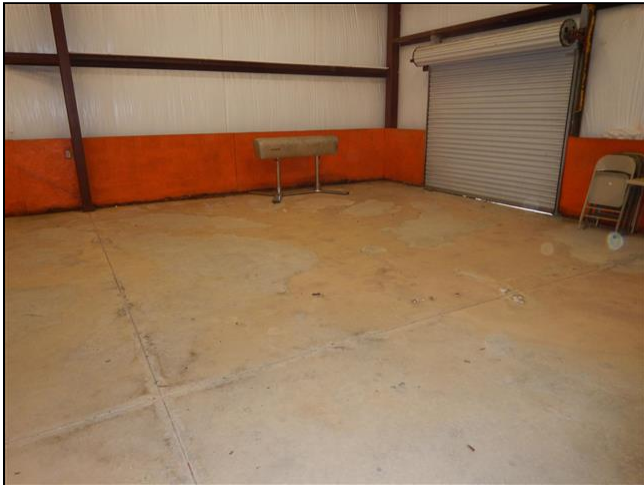
4.0 Item 1(Picture) Water is leaking into the building under the wall due to poor landscaping.
