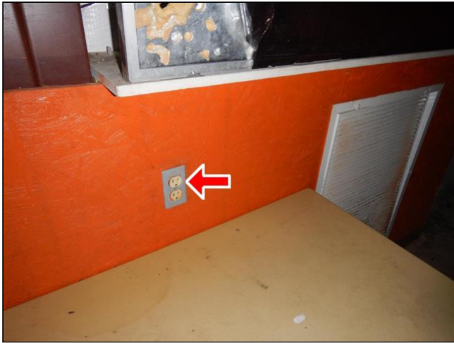
Item 8 - Item 1(Picture) This receptacle did not have power.
