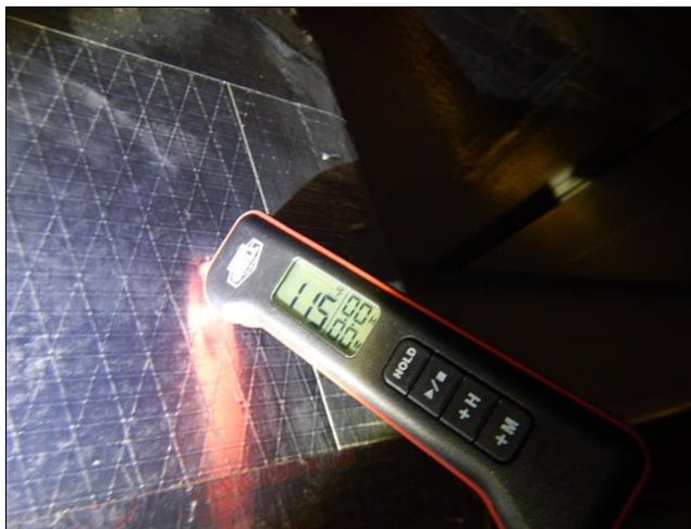
7.0 Item 2(Picture) The HVAC for the office area was pulling in 80 degree air and heating to 115 degrees. This is a normal operating temperature range.
