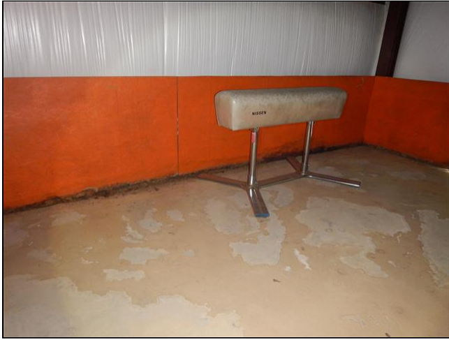
3.1 Item 1(Picture) The plywood walls in the gym has water damage.
