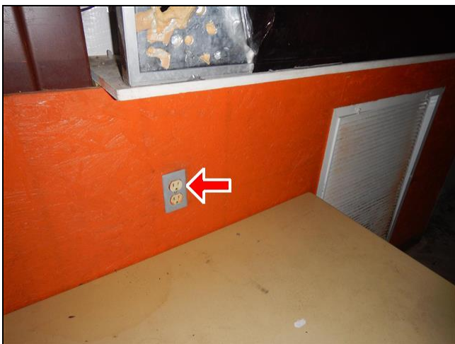
6.2 Item 1(Picture) This receptacle did not have power.
