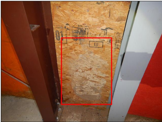
Item 7 - Item 1(Picture) Termites have been in this wall area in the gym. Recommend a qualified contractor to evaluate and repair as necessary.
