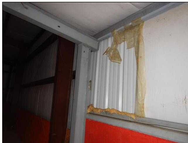
Item 12 - Item 2(Picture) The wall insulation is damaged or missing in several areas.
