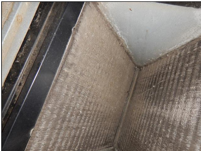
7.3 Item 3(Picture) The coil in the air handler is very dirty.
