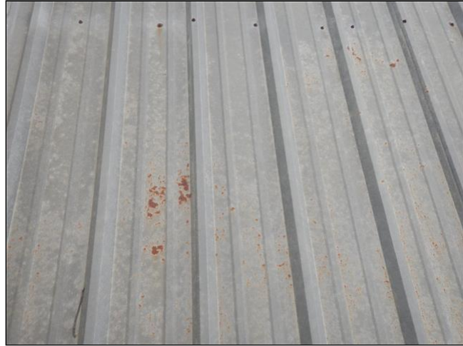
Item 1 - Item 2(Picture) There is rust on several pieces of roofing. The rust needs to be sanded and painted.
