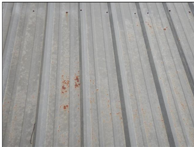
1.0 Item 2(Picture) There is rust on several pieces of roofing. The rust needs to be sanded and painted.
