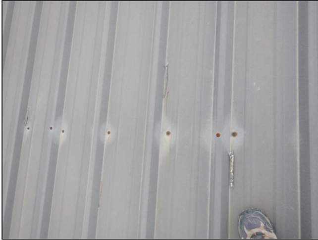
Item 1 - Item 1(Picture) The screws for the roofing are corroded with rust. They are recommended to be replaced.
