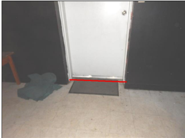
Item 2 - Item 2(Picture) Water and air is leaking around the exterior doors.
