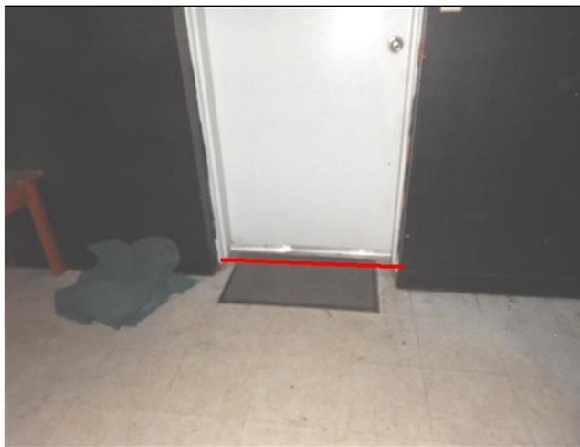
2.1 Item 2(Picture) Water and air is leaking around the exterior doors.
