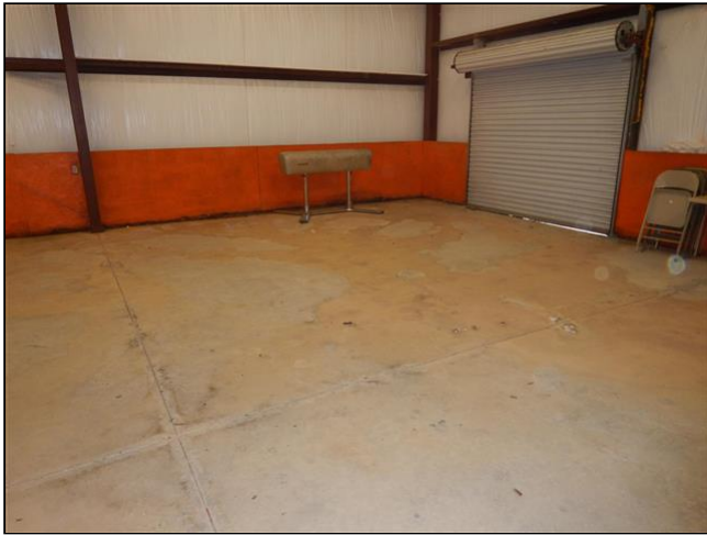
Item 6 - Item 1(Picture) Water is leaking into the building under the wall due to poor landscaping.
