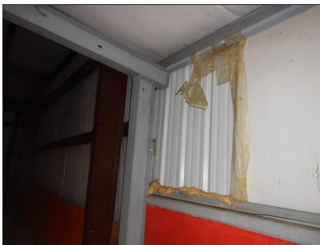
8.0 Item 2(Picture) The wall insulation is damaged or missing in several areas.
